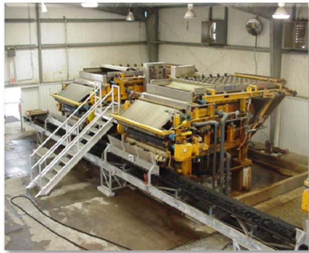
Bio-solids dewatering equipment
