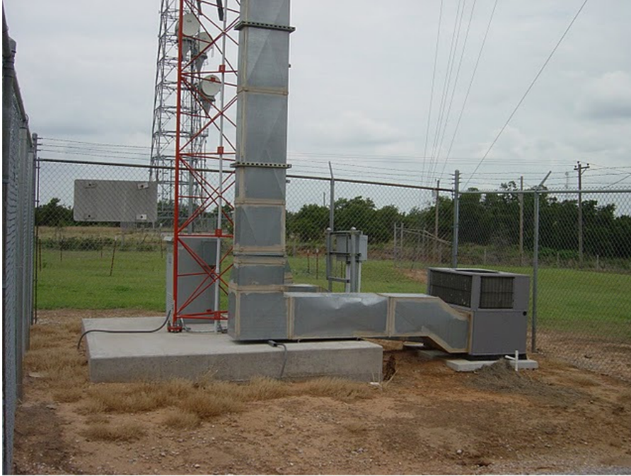
Figure 10 - HVAC unit, Ductwork, Security fence
