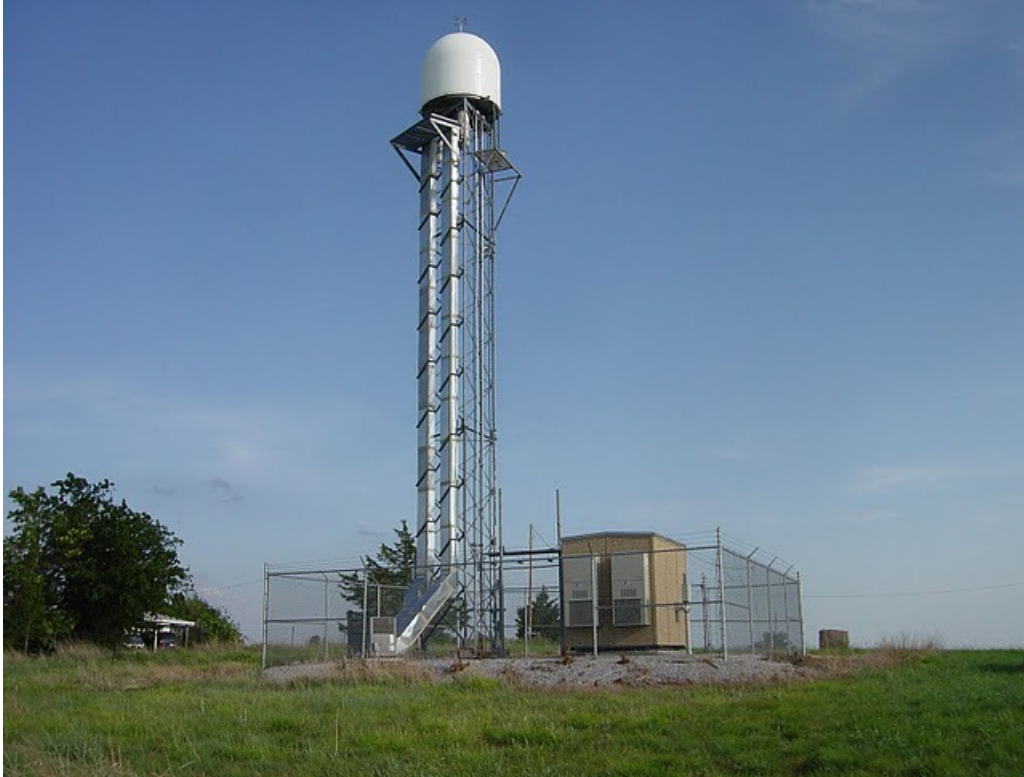
Figure 30 - Complete tall tower installation with prefabricated shed
