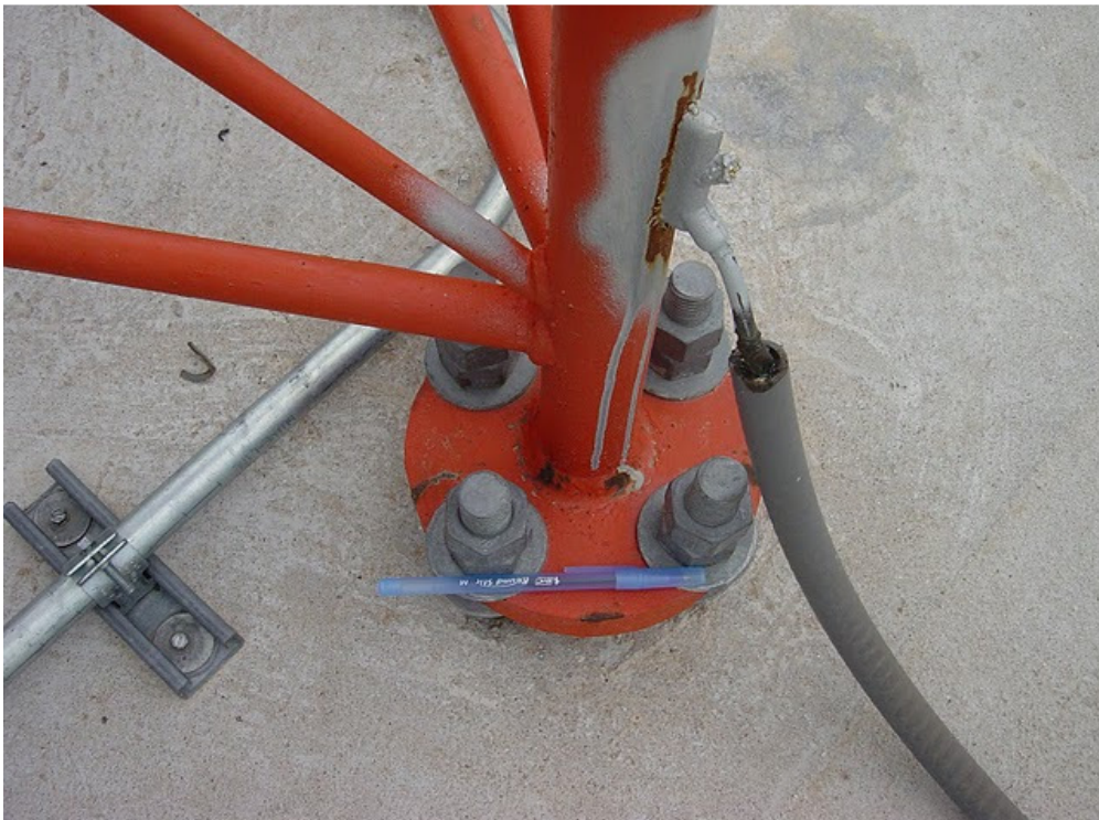
Figure 6 - Top view tower anchoring with grounding cable visible
