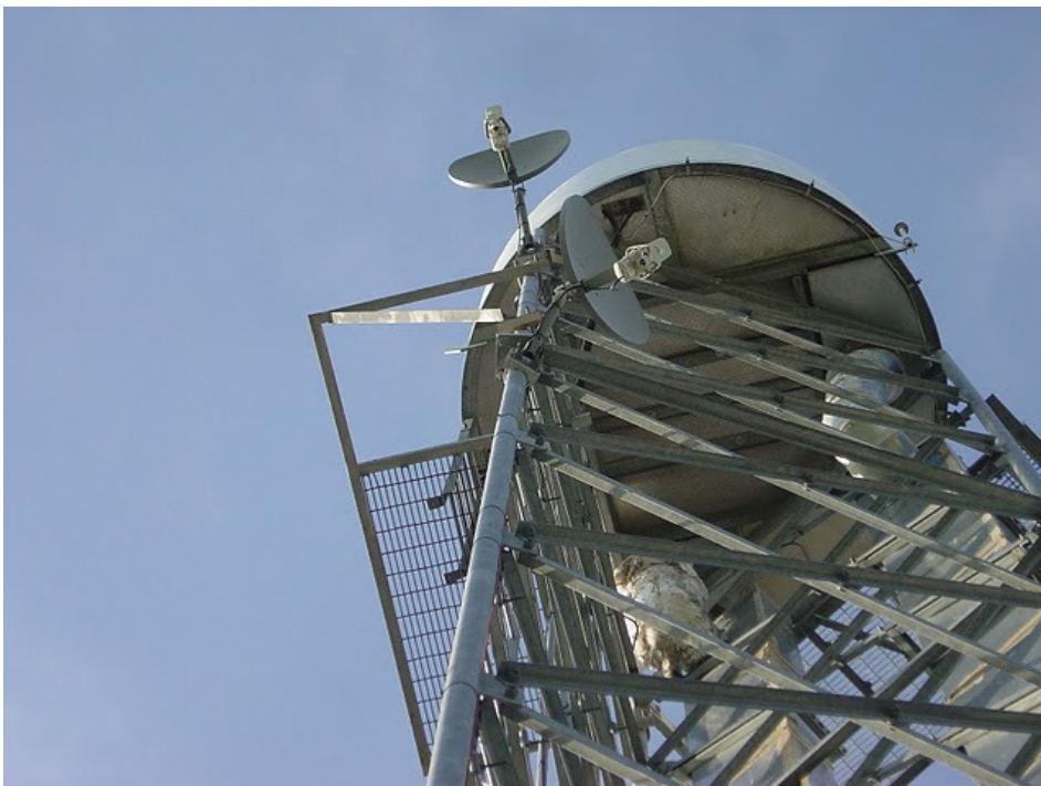
Figure 23 - Wireless radio antennas mounted to tower
