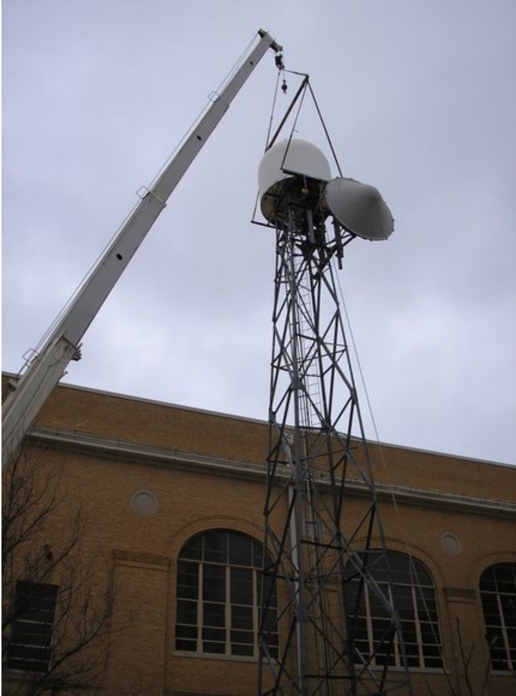
Figure 17 - A square pyramid tower adjacent to an existing building with a microwave antenna mounted alongside for communications.
