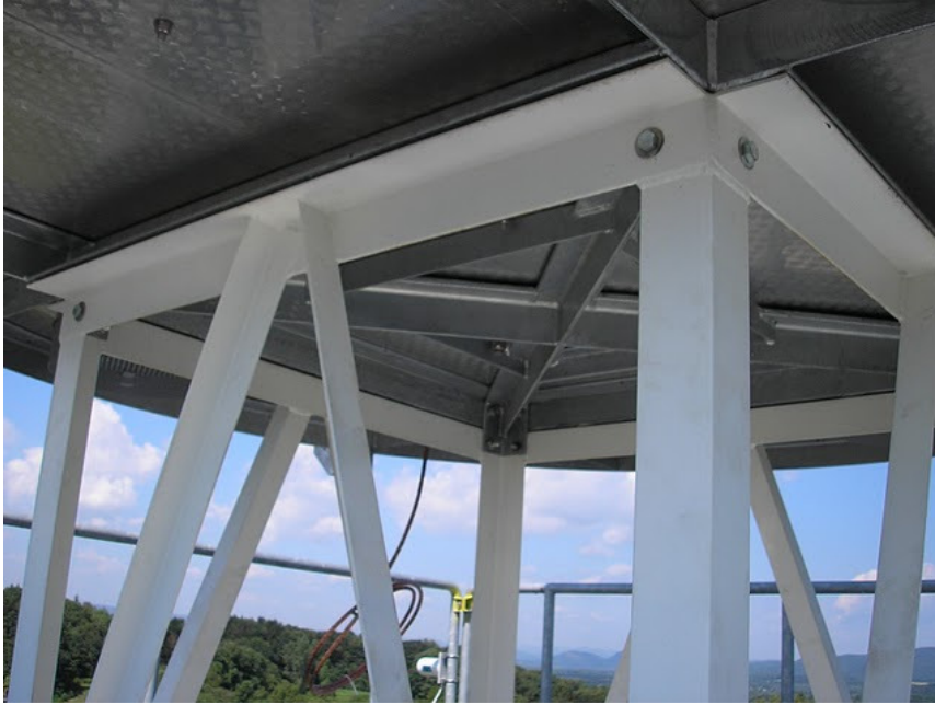
Figure 20 - Radar mount elevated off the platform
