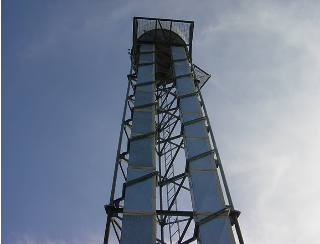
Figure 22 - Outgoing and return insulated metal duct with booster fans strapped to tower for ground HVAC installation
