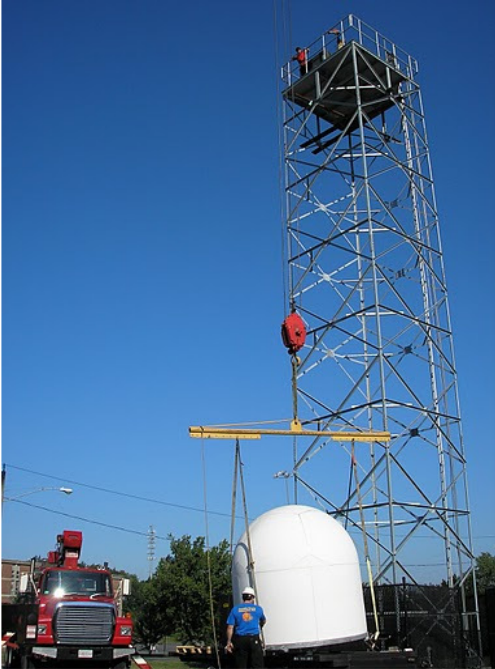
Figure 19 - Radar is craned onto a platform constructed at the top of the square tower
