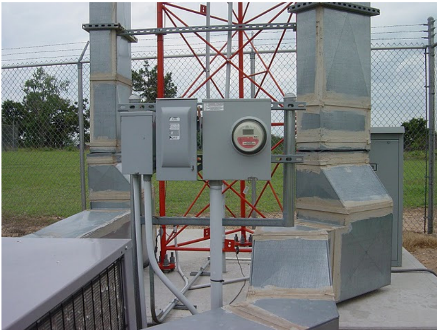
Figure 11 - Breaker box, Meter, Ductwork
