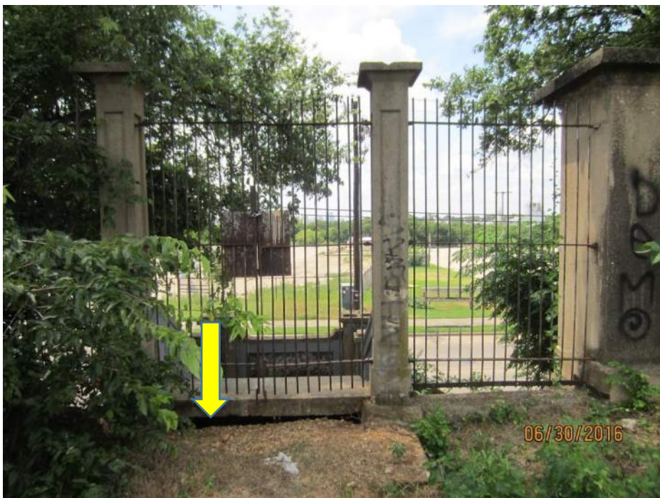
Photograph 40 – Large void under grand stairway
