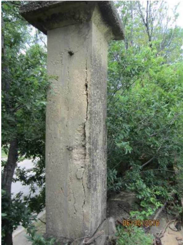
Photograph 29 – Cracked, spalled and hollow-sounding concrete on large column, upper wall
