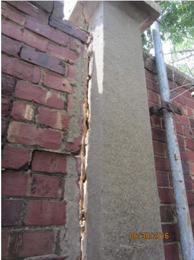
Photograph 33 – Significant vertical gap in wall, southeast corner
