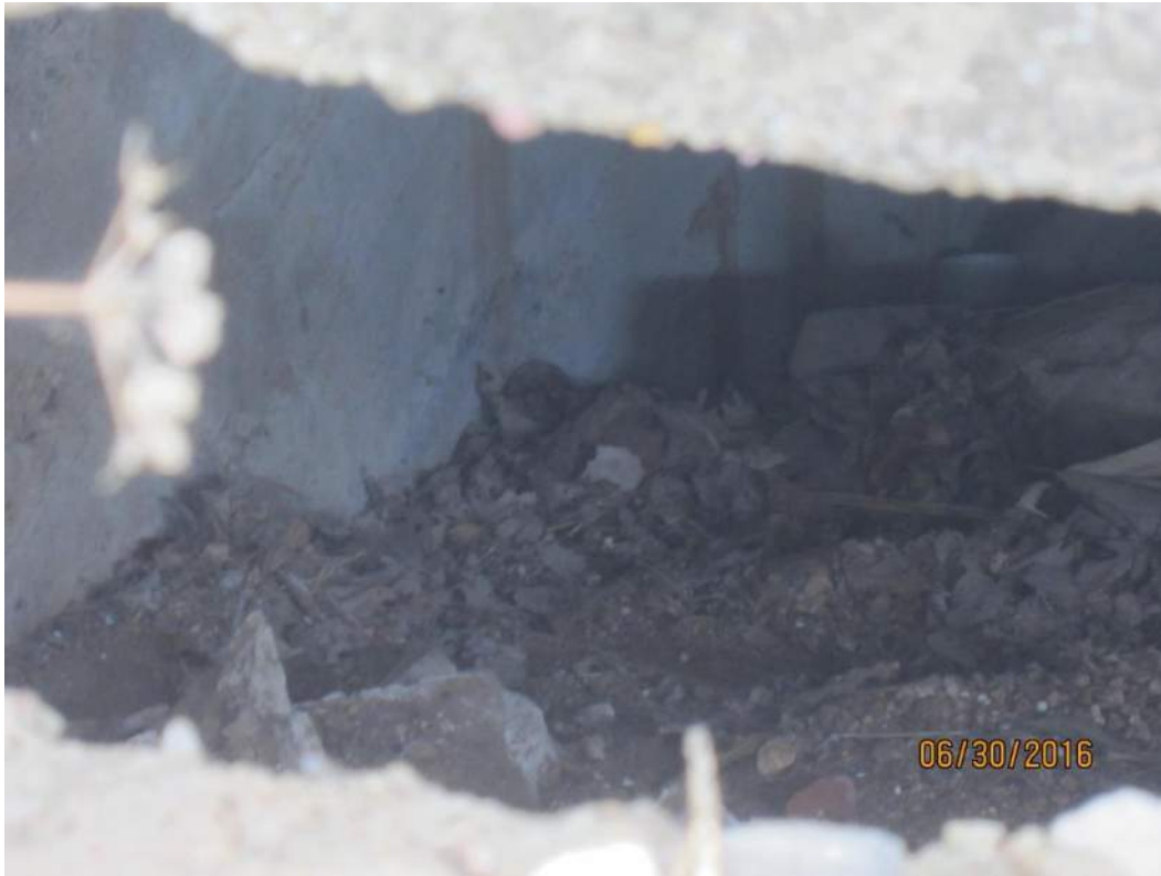
Photograph 41 – Large void under grand stairway
