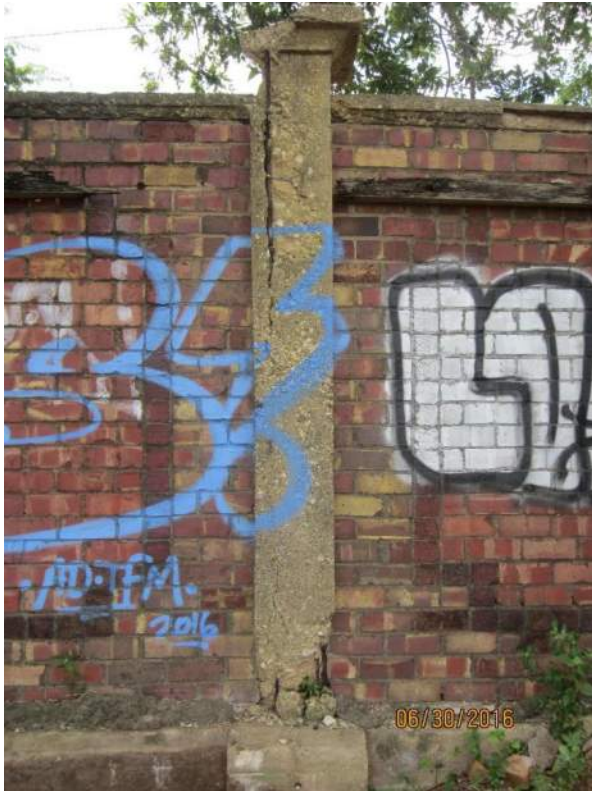
Photograph 25 – Vertical cracks, spalls, and hollow sounding concrete on columns at upper wall
