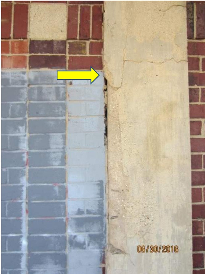
Photograph 5 – Spalled concrete at pilaster shows brick keyway
