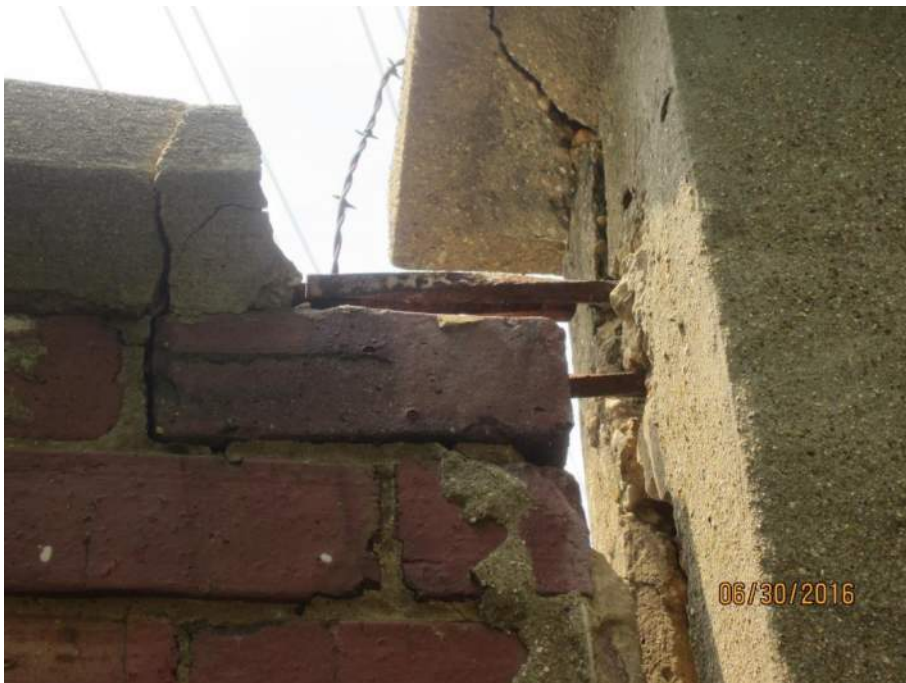
Photograph 34 – Significant vertical gap in wall, southeast corner
