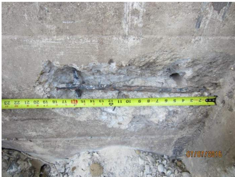
Photograph 16 – Twisted steel reinforcing in lower section of backup wall
