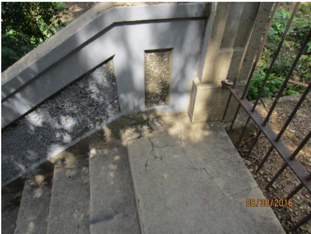
Photograph 38 – Cracked and spalled concrete topping at grand stairway
