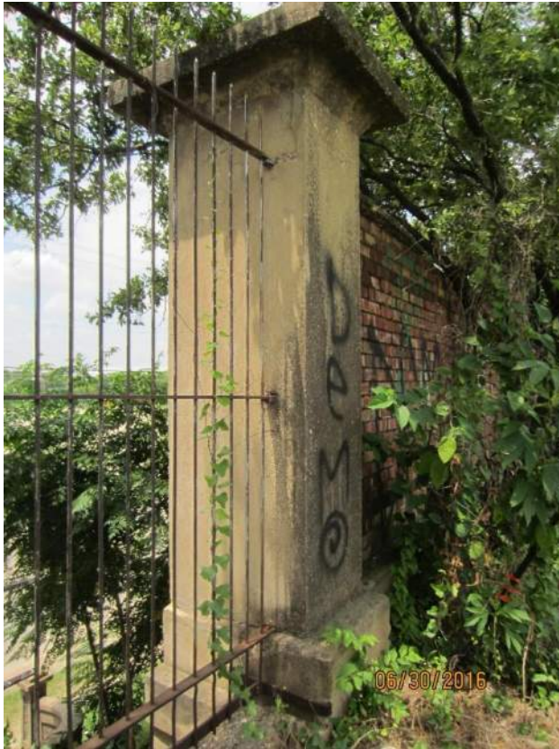
Photograph 9 – Iron fence section in lieu of single wythe brick masonry at upper section of wall
