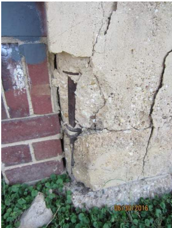
Photograph 18 – Cracked, delaminated and spalled concrete at pilaster, lower wall
