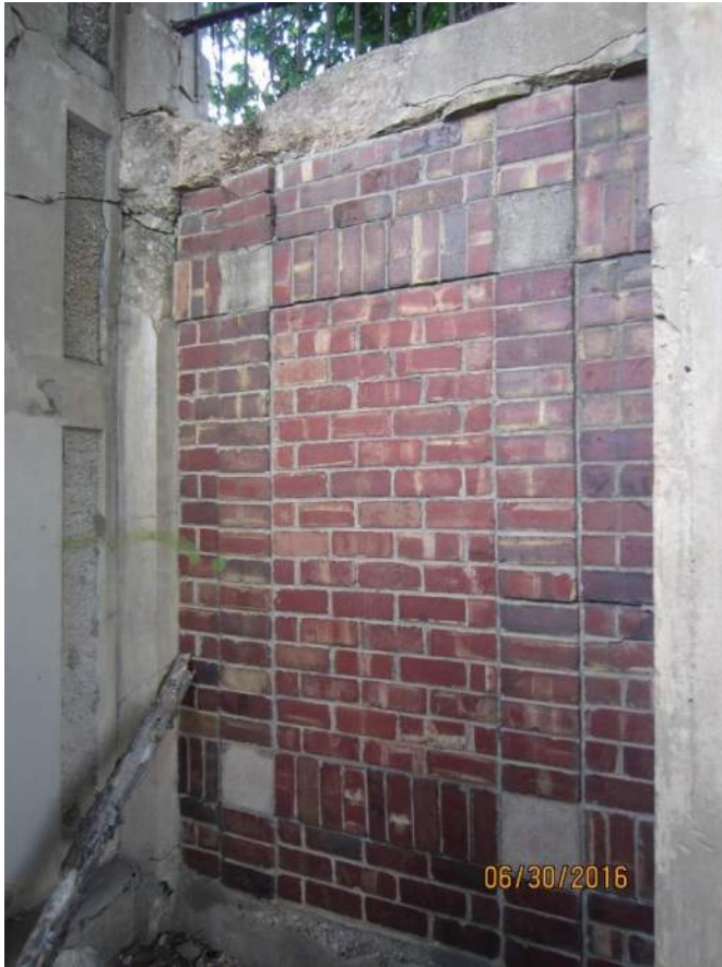
Photograph 39 – Cracked and spalled concrete and brick, east side of grand stairway
