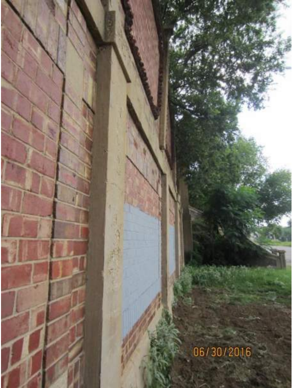
Photograph 11 – Wall leans to the south (right)
