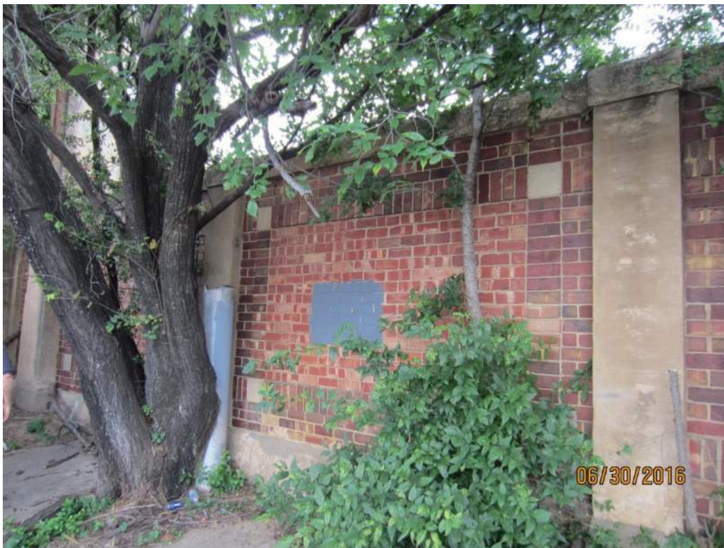
Photograph 44 – Large tree at base of wall, south side
