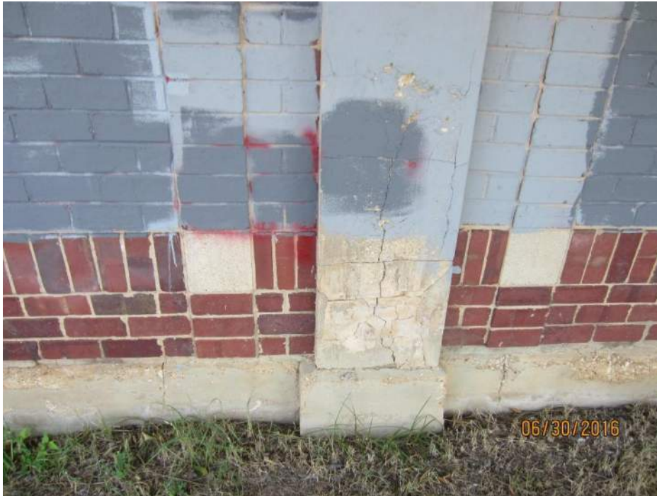
Photograph 19 – Cracked and hollow-sounding concrete on pilaster, lower wall
