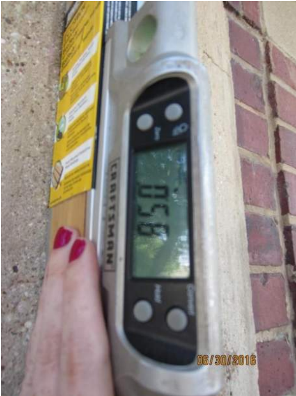
Photograph 11 – Lower pilaster 5 degrees out of plumb
