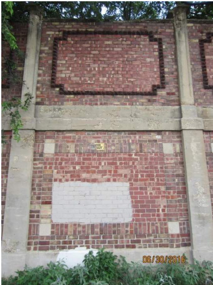
Photograph 4 – Concrete pilasters separate the brick panels on lower section of wall; concrete columns separate brick panels on upper section
