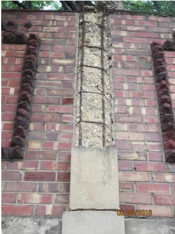
Photograph 17 – Spalled concrete and exposed reinforcing on south face at upper column; note missing concrete cap on top of wall
