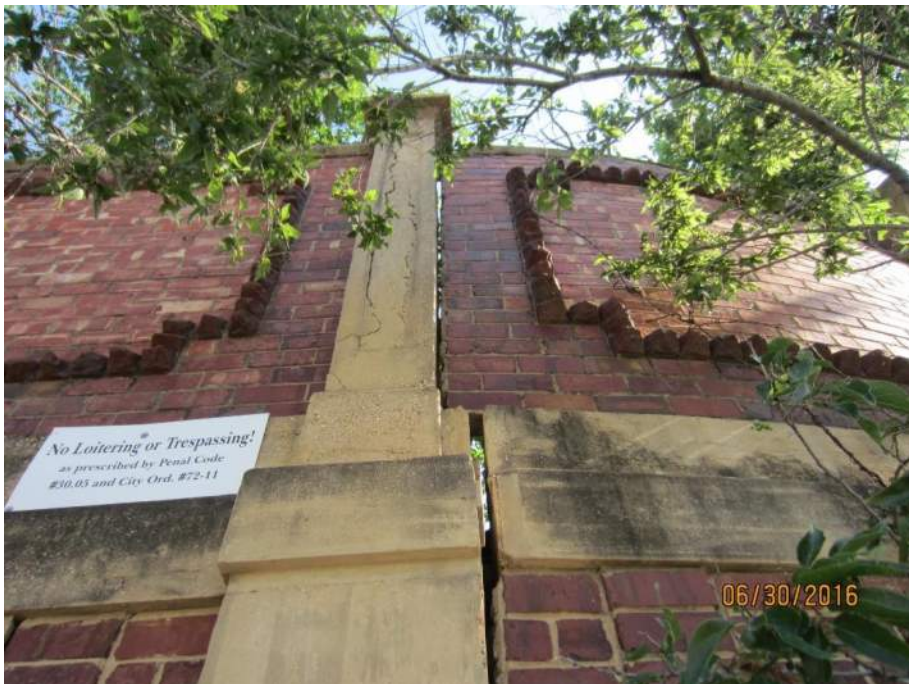
Photograph 32 – Significant vertical gap in wall, southeast corner
