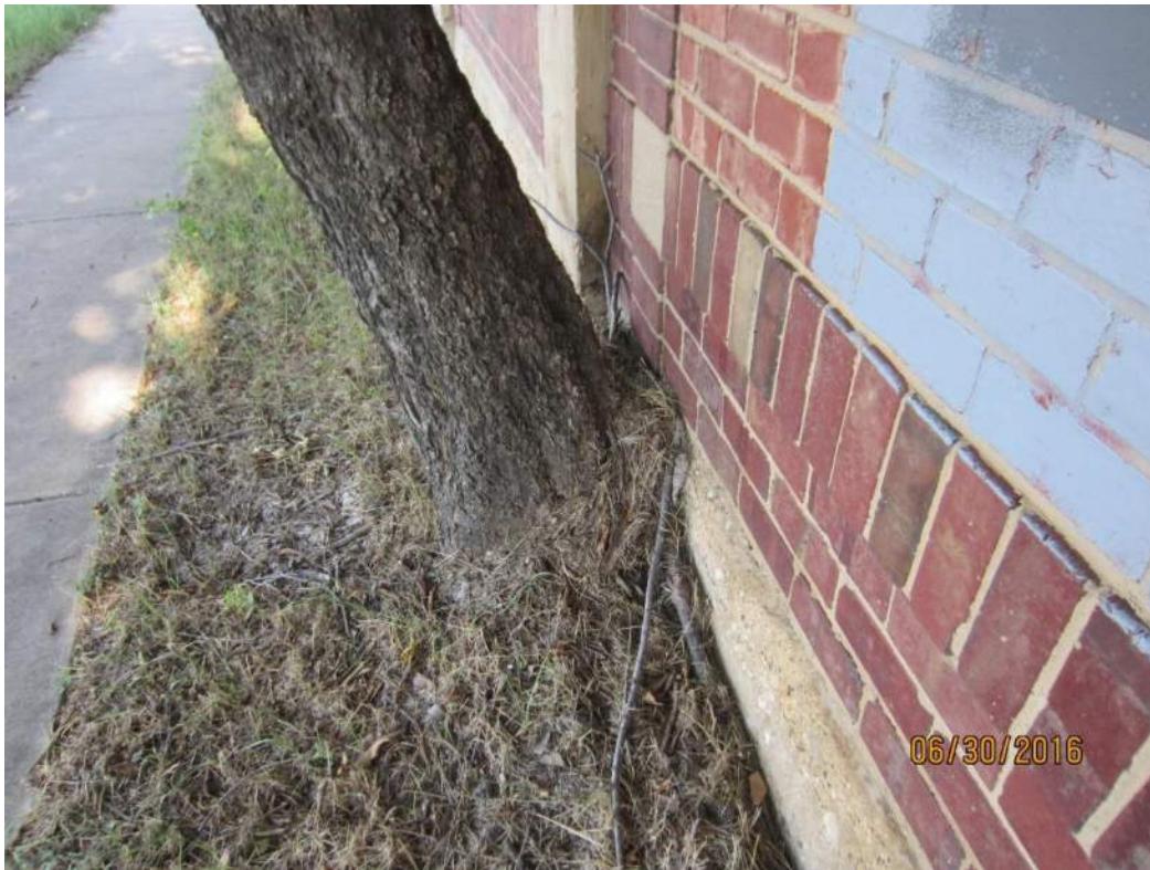
Photograph 43 – Large tree at base of wall, south side
