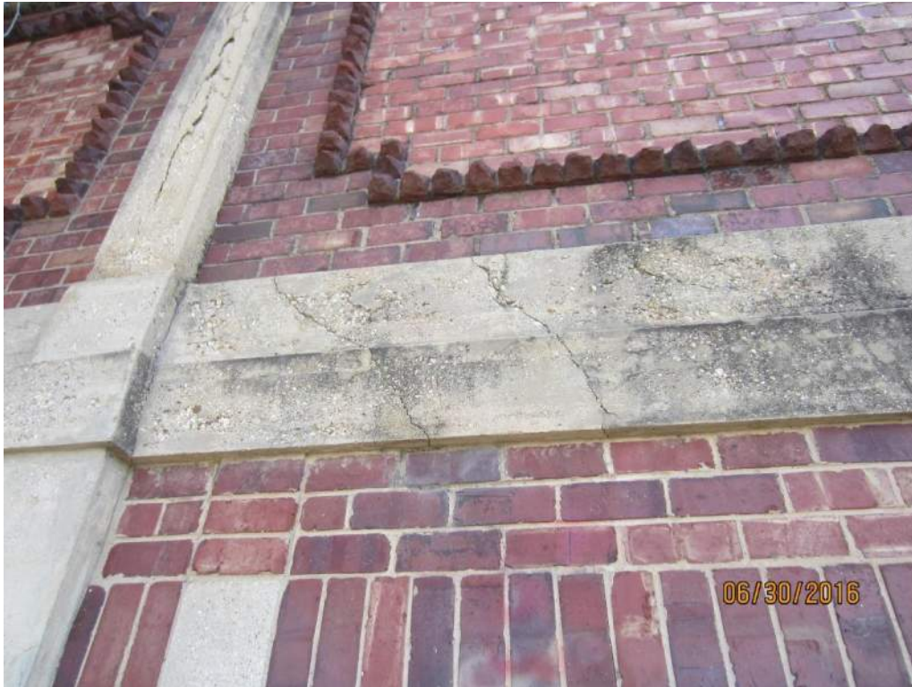
Photograph 21 – Cracks in concrete beams between upper and lower sections of wall; note cracks and delaminated concrete in upper column
