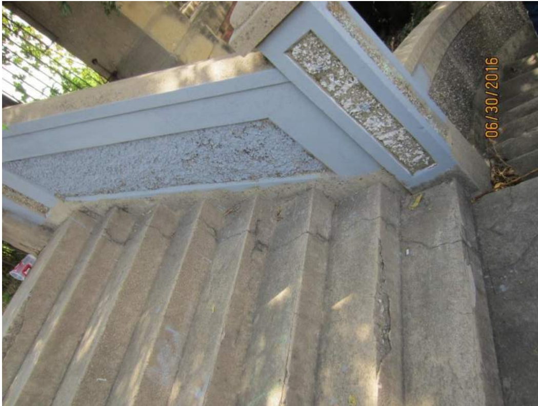
Photograph 37 – Cracks in concrete steps and risers parallel to sidewalls
