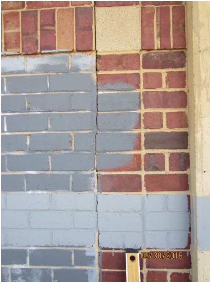
Photograph 31 – Crack in mortar joint at brick veneer, lower wall
