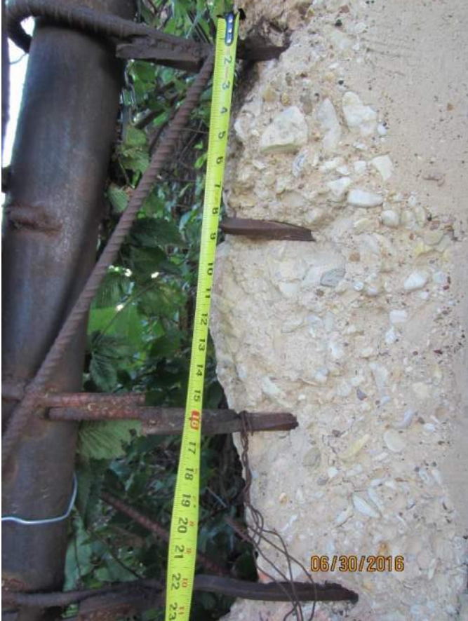
Photograph 13 – Twisted reinforcing steel in lower backup wall
