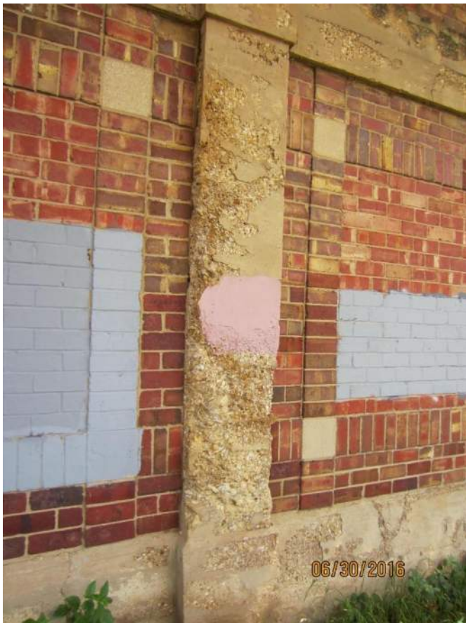
Photograph 20 – Spalled face of pilaster, lower wall
