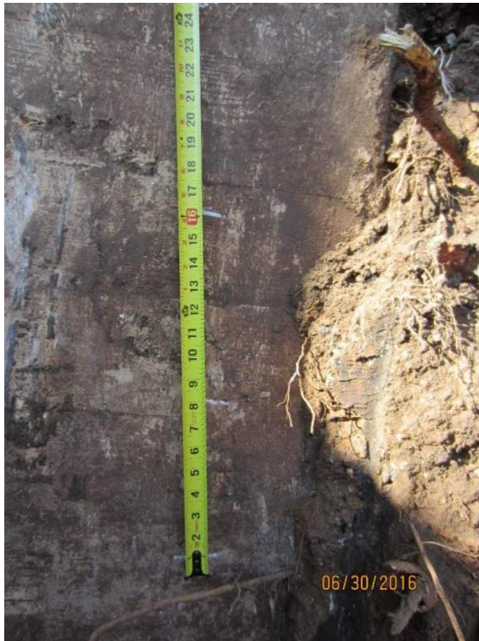
Photograph 15 – Horizontal steel detected in pilaster on back side of lower section of wall
