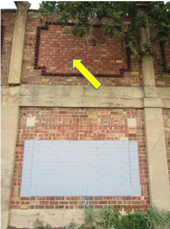
Photograph 36 – Diagonal crack in upper masonry wall
