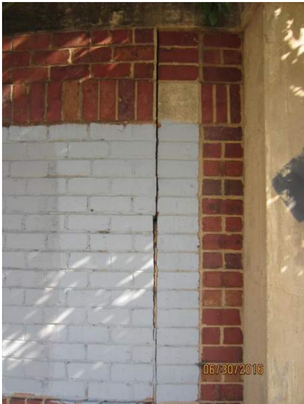
Photograph 30 – Cracked and open mortar joint at brick veneer, lower wall
