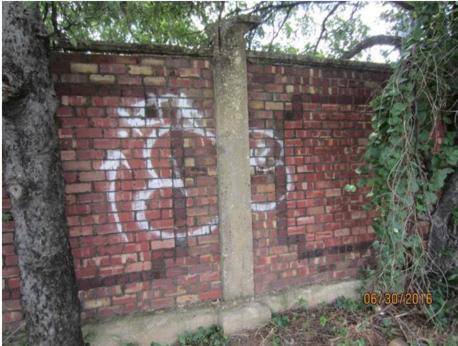
Photograph 27 – Broken column capital and severely deteriorated coping on top of brick wall
