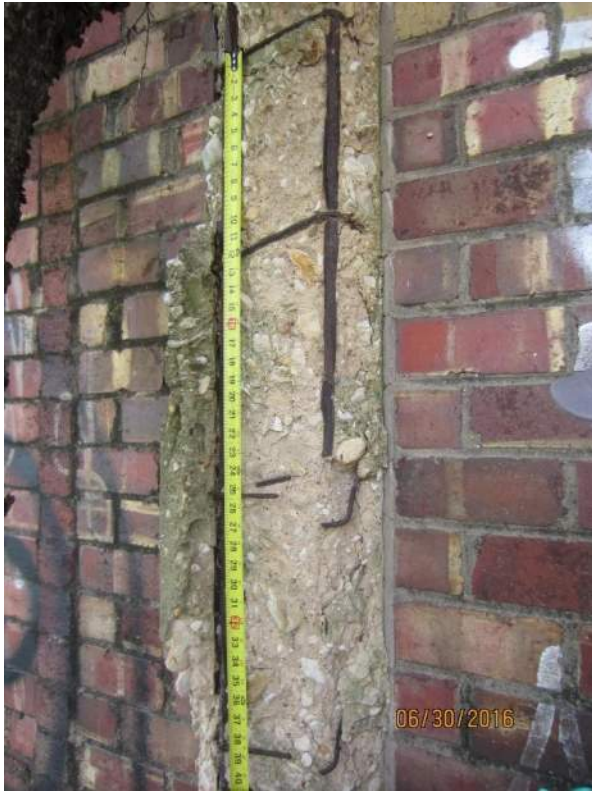
Photograph 23 – Spalled concrete and exposed reinforcing steel on back side of upper column
